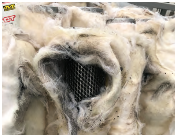
Figure 12 Coalescer Element Failure
