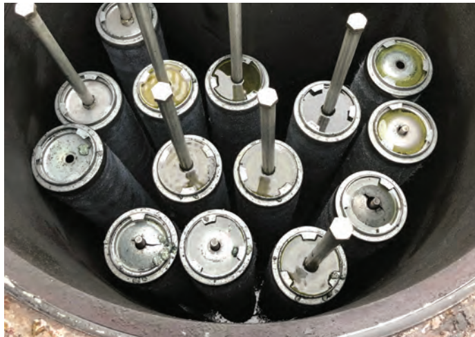
Figure 3 Damaged Coalescing Elements Demonstrating Bypass
