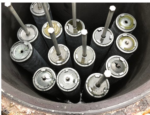
Figure 12 Coalescer Element Failure
